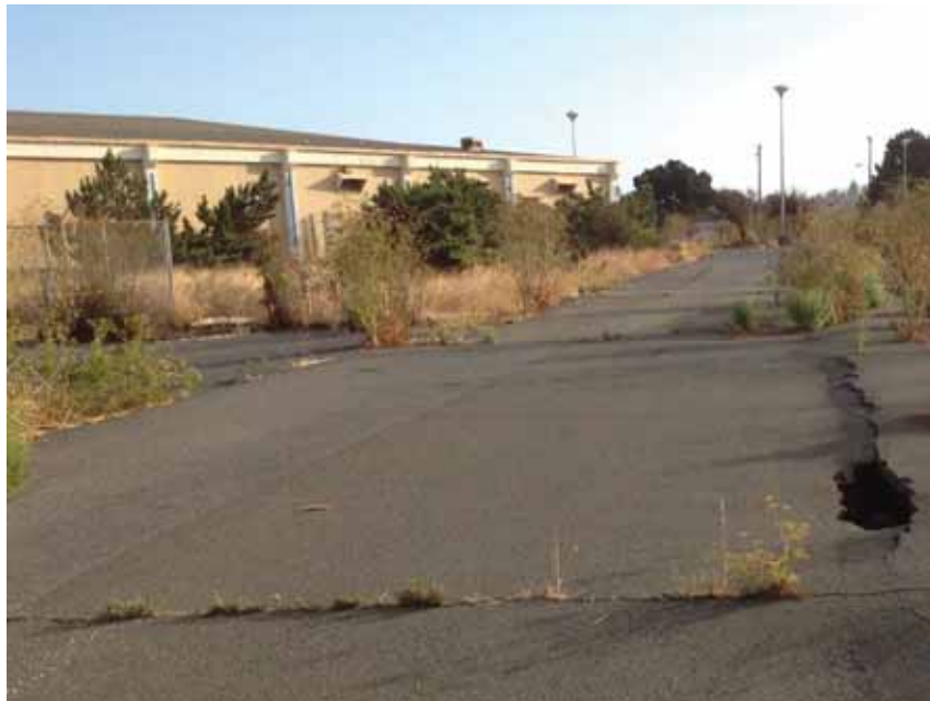
Photograph 2 Settlement induced damage and visible void adjacent to duct bank near south west corner of site. (10/06/2015)
