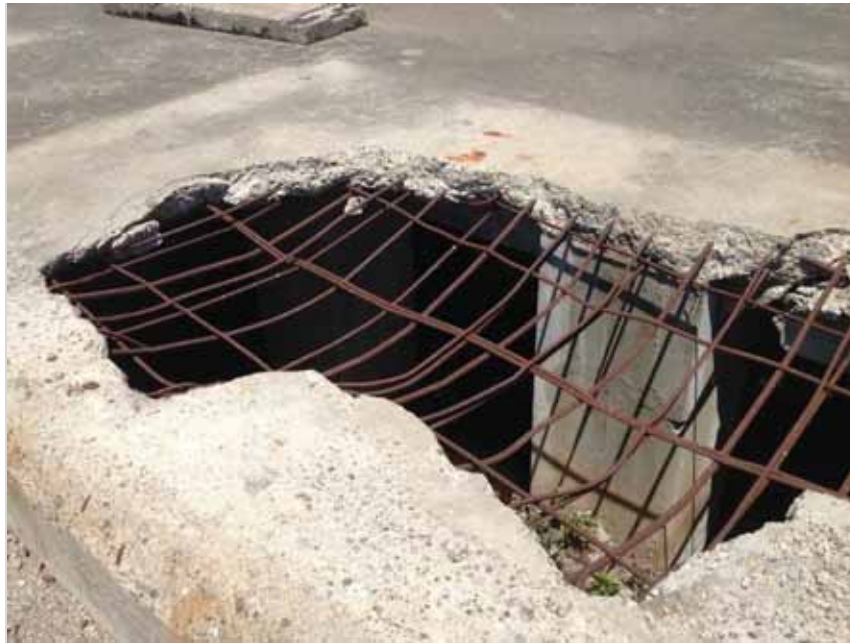
Photograph 1 Foundation and visible void near Mare Island Strait. (05/18/2015)
