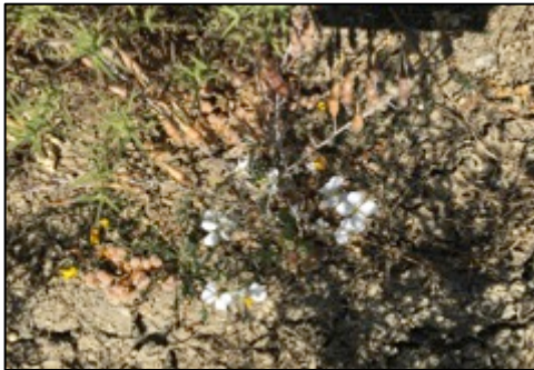
SWL-4. Minor soil surface cracking can be seen in the photo, evidence of ponding.
