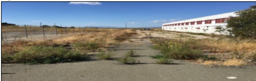
SWL-31. Ponded concrete basin that has “in-floor” ~2’x2’ drainage grate with cattails growing out of it.
