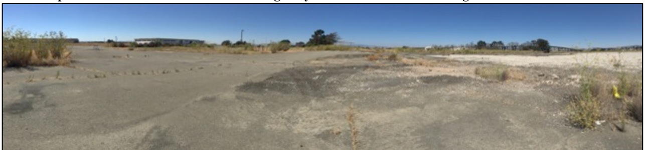
Eroding asphalt areas with little to no vegetation growing through.
