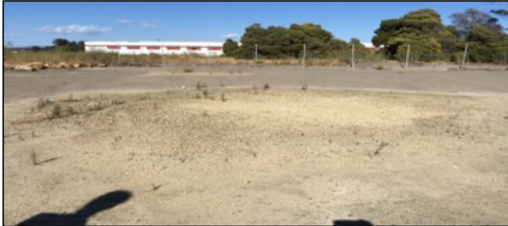
SWL-17. Isolated, ponded hardscape over pavement. Recommend discounting this area.
