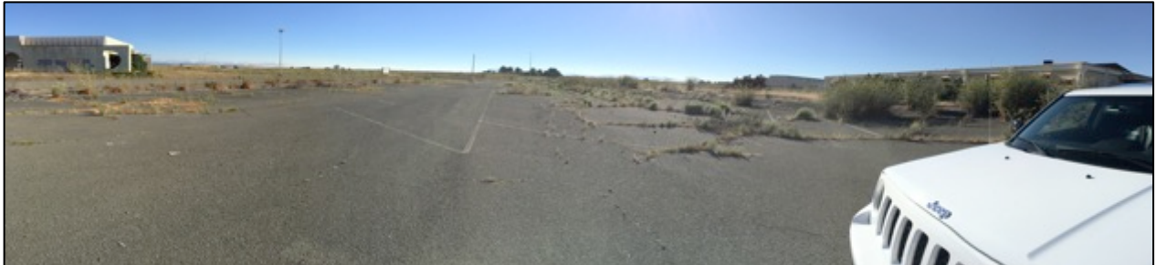
Extensive eroding asphalt with some ruderal upland vegetation growing through.
