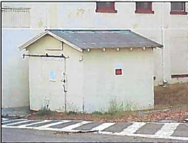
E – Small Industrial Garage/ Shed/ Pumhouse/ Electrical Facility (Building 1278, adjacent to H081)
