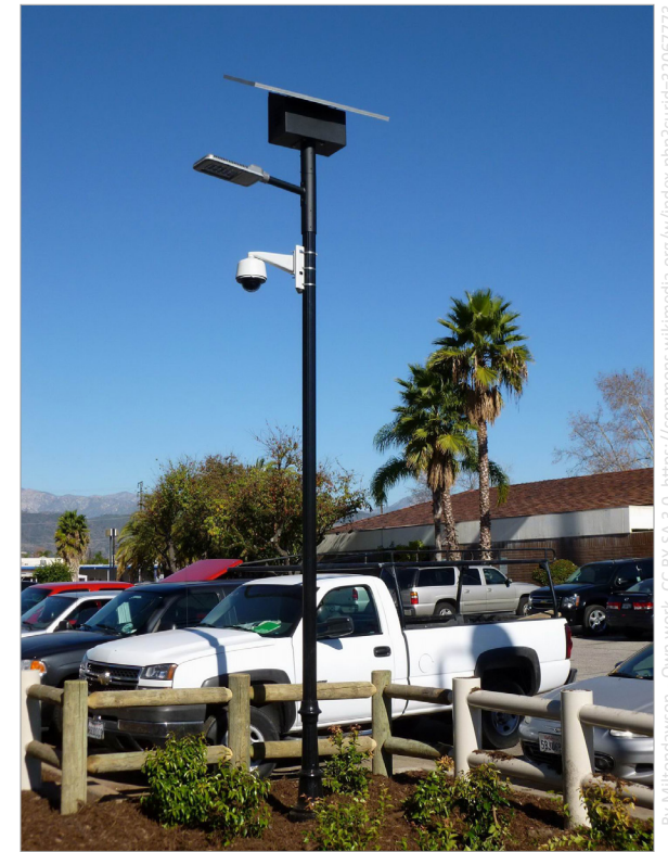
Solar powered light located in a landscaped area within a parking lot.
