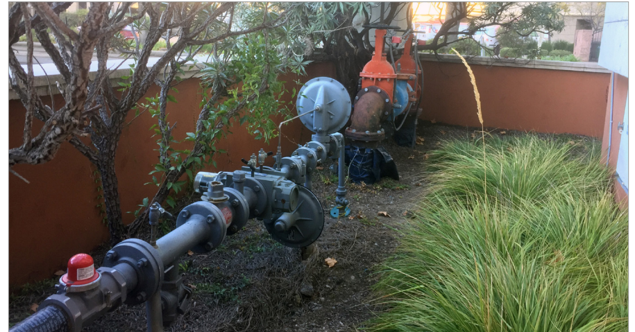
Back : Ground mechanical equipment is screened from view with landscaping and a knee wall.
