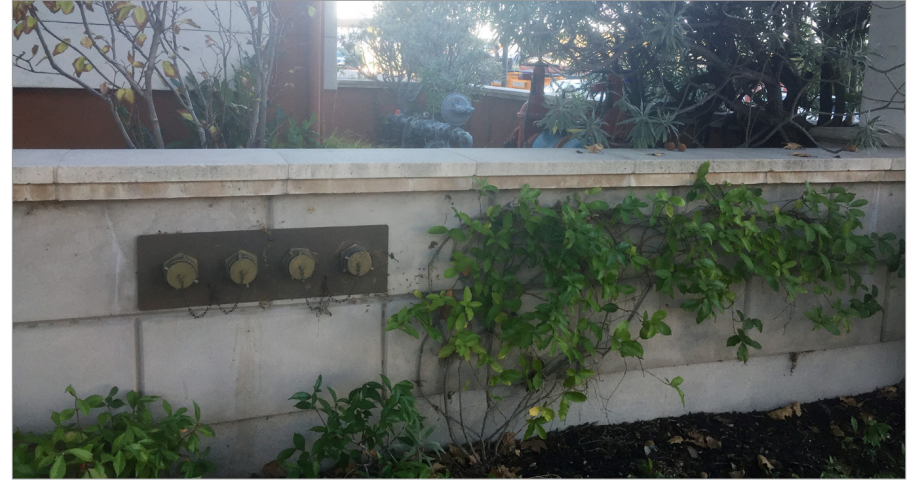
Front : Concrete block knee wall used to screen ground mechanical equipment.
