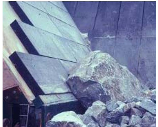
Primary feed hopper lined with Trellex Wear resistant elements type PP.
